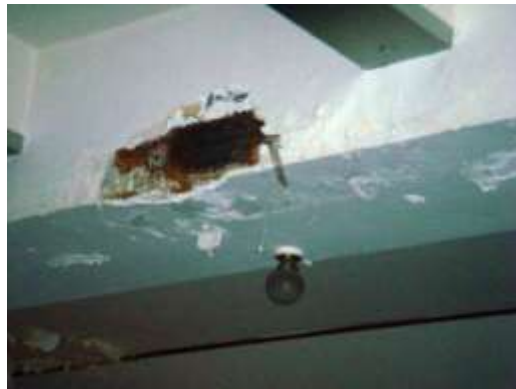
Unused for many years, the ballroom is in serious disrepair.
